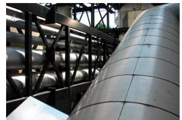
Pictures from the Waste Incineration plant "I/S Vestforbrændingen" for a Heat Recovery project based on Flue Gas Scrubbers with Heat Pumps boosting Water Temperature for District Heating usage.
